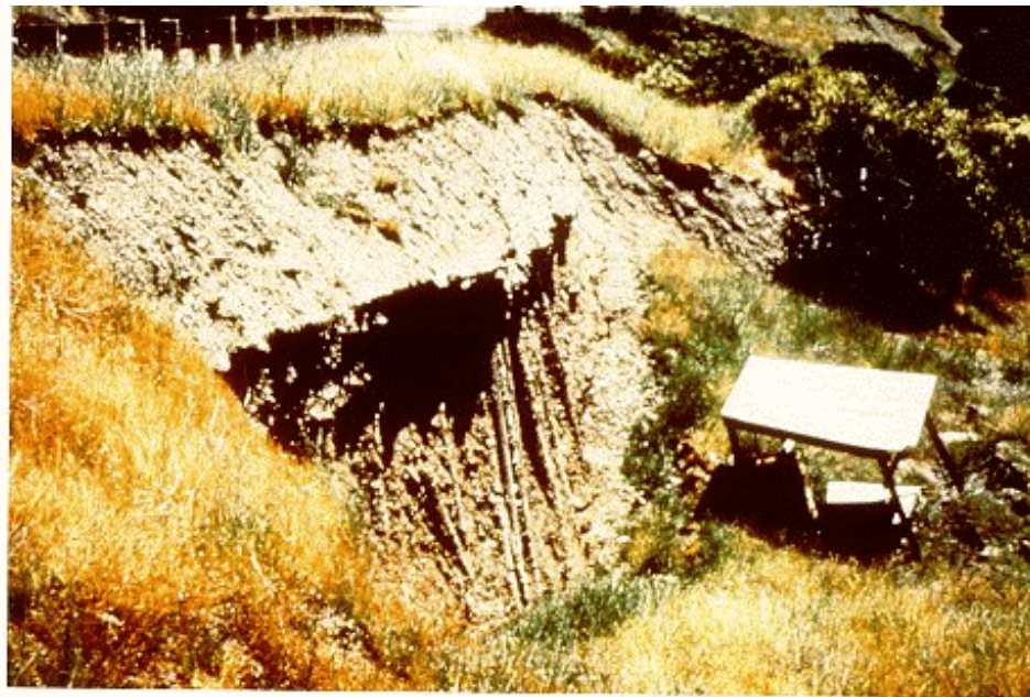
Figure 3-13. Photo of Slope Stabilization at FH-7 Project in Mendocino National Forest, California.
