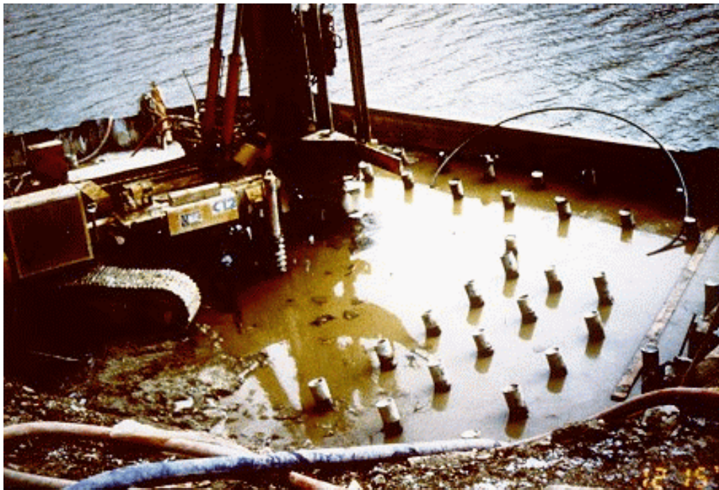
Figure 3-4. Micropiles Used Under New Abutments for Bridge Over Mahoning Creek, Armstrong County, PA (after Pearlman and Wolosick, 1992).
